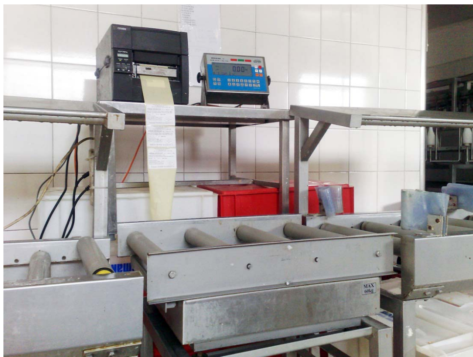
Fig. 66 Labelling system installed on carcasses partition line
